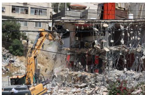
An Israeli excavator demolishes 2-storey building, belonging to Palestinian al-Rajbi family, claiming that they are "unlicensed" in Silwan Neighbourhood of East Jerusalem, Jerusalem on May 10, 2022. Mostafa Alkharouf - Anadolu Agency
